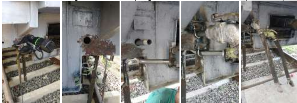
Modification in steps: Hole cutting by Magnetic drilling M/c, Metal Pipe and air hose fitment
