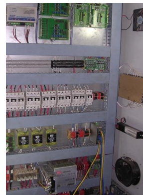
Data acquisition panel
